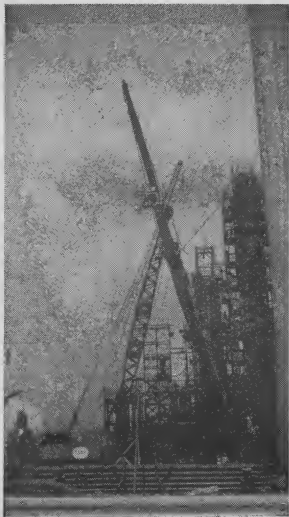
Giants cooperate as a crane raises a derrick into position at No. 9 Visbreaker for some really heavy lifting. For other pictures of the major job done at No. 9, see page 4.
